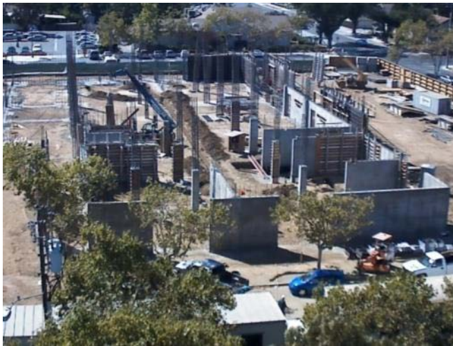
View captured by the Library Construction Cam, accessible to the public via the City website.
