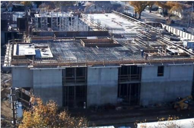
View captured by the Library Construction Cam in early December, accessible to the public via the City website.
